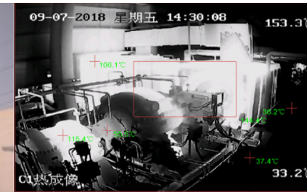
A high-value compressor is being monitored by thermal temperature sensing
