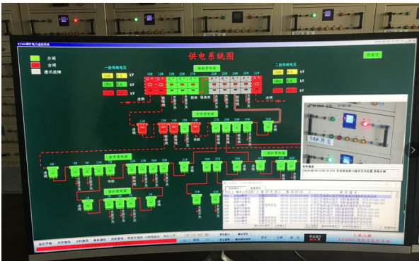
A electrical integrators' platform
